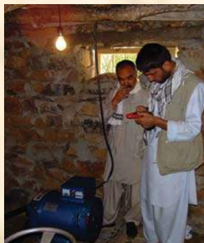
Afghanistan national workers checking generating equipment.
